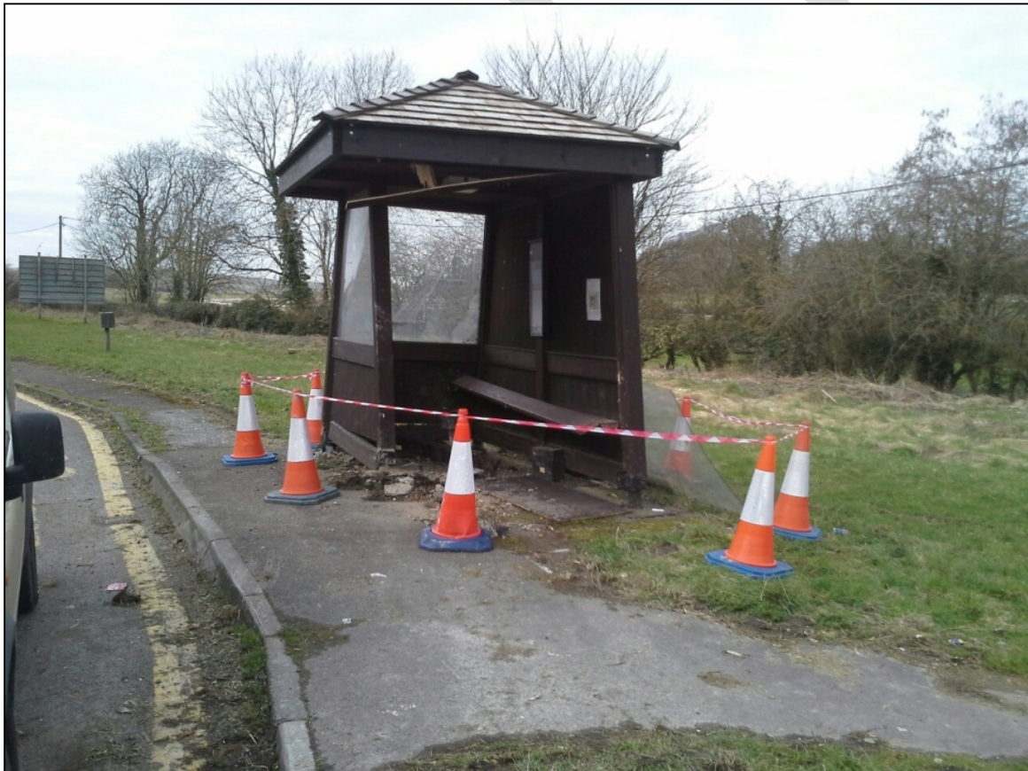
Street furniture structural damage (DAST)
