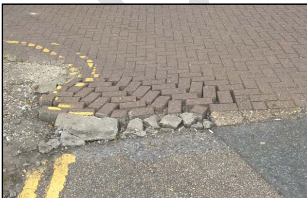
Footway trip, slab profile/rocking slab (SLPF)
