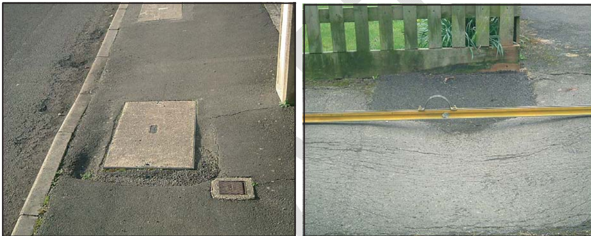
Depressions in footway (DEPR)
