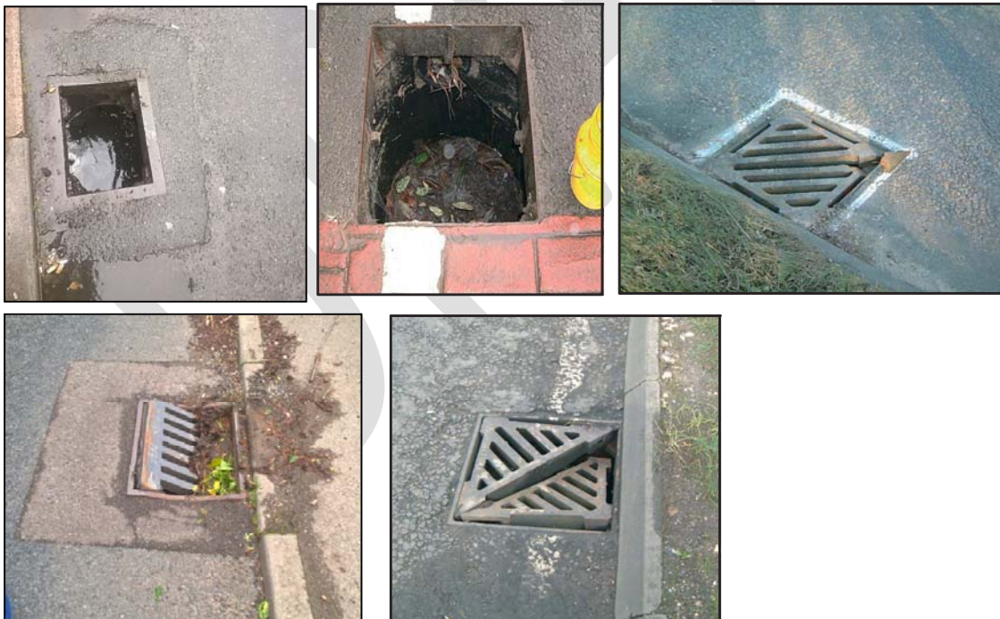
Cracked, missing, broken or level difference (IBCK, MISS, IDLV, LEVE)
